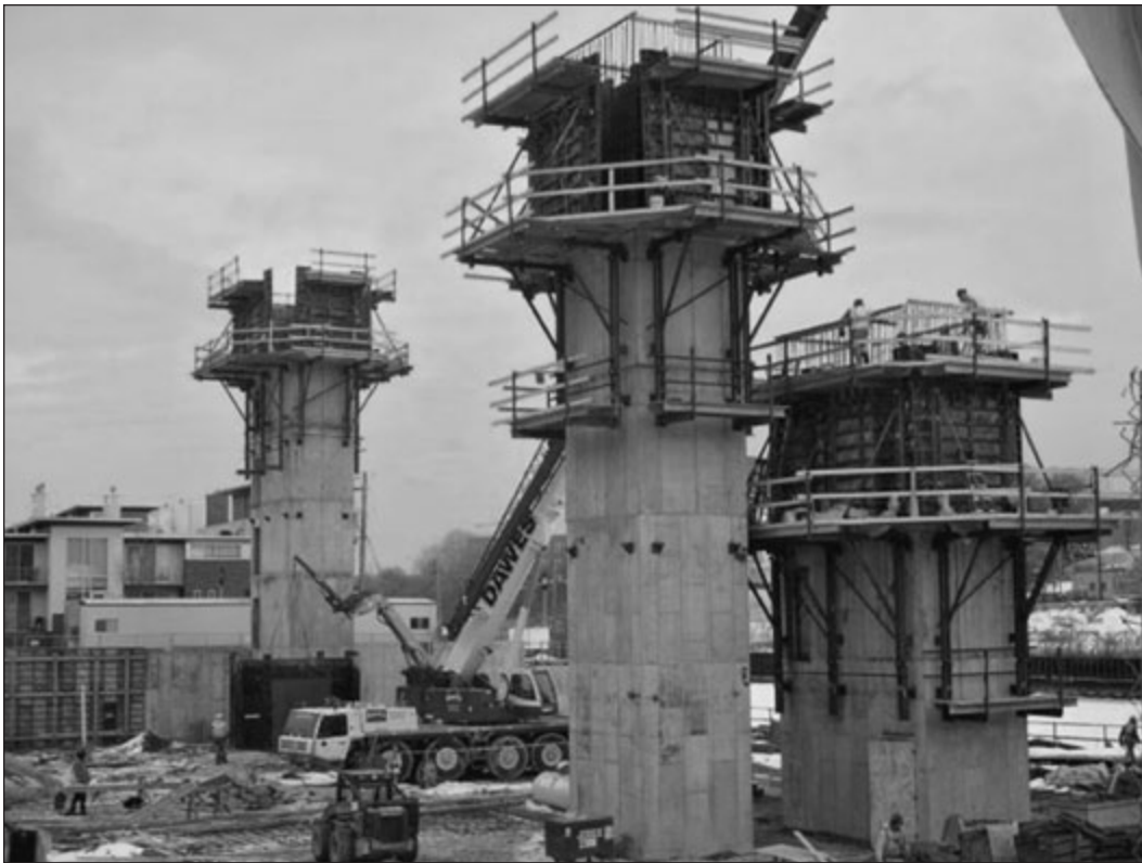
This Space-Lift™ concrete jump forming system integrates the forming system and work platforms. The workers do not need to be on the platform when the forms are being jumped, which increases safety. Photo courtesy: Symons.
