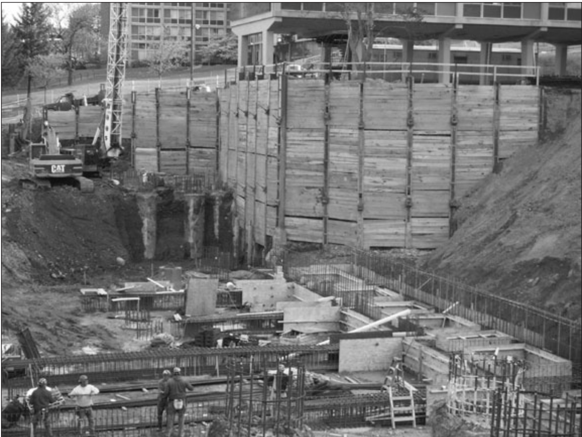
This soldier pile and lagging retention system was installed by Hayward Baker for construction of the Ernie Davis Hall at Syracuse University in Syracuse, New York. The steel H-sections are driven into the unexcavated earth along the planned excavation limits. Timber lagging is placed between the piles as the excavation progresses. Steel tiebacks through the H-sections into the earth are installed at planned intervals to resist the pressure of the retained earth. The open work area permits rapid excavation and installation of the structure that can produce both cost savings and schedule acceleration. This type of retention system can be installed in many soil types. Photo courtesy of Hayward Baker Inc.
